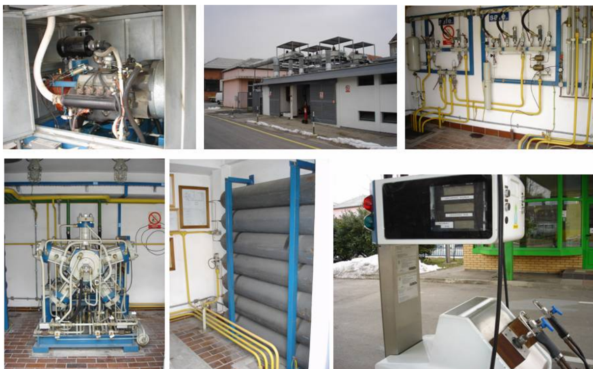
Figure 26. Details of existing CNG filling station (location: Radnička cesta 1)
